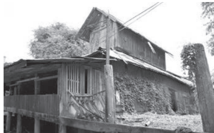
Fig.3.75. Deterioration of Thin-Gaza Kyaung* 5
