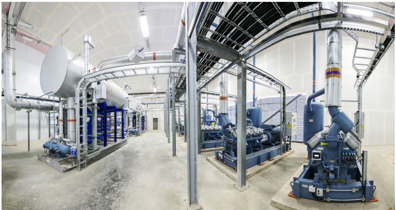
Fig. 9: GEA Piston Compressor Packages at a Processing Facility. Source: GEA Industrial Refrigeration Solutions[51]
