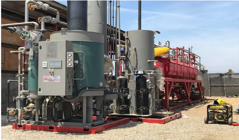
Figure 3.4:Overall View of Thermo-vacuum Drying System Installed.
