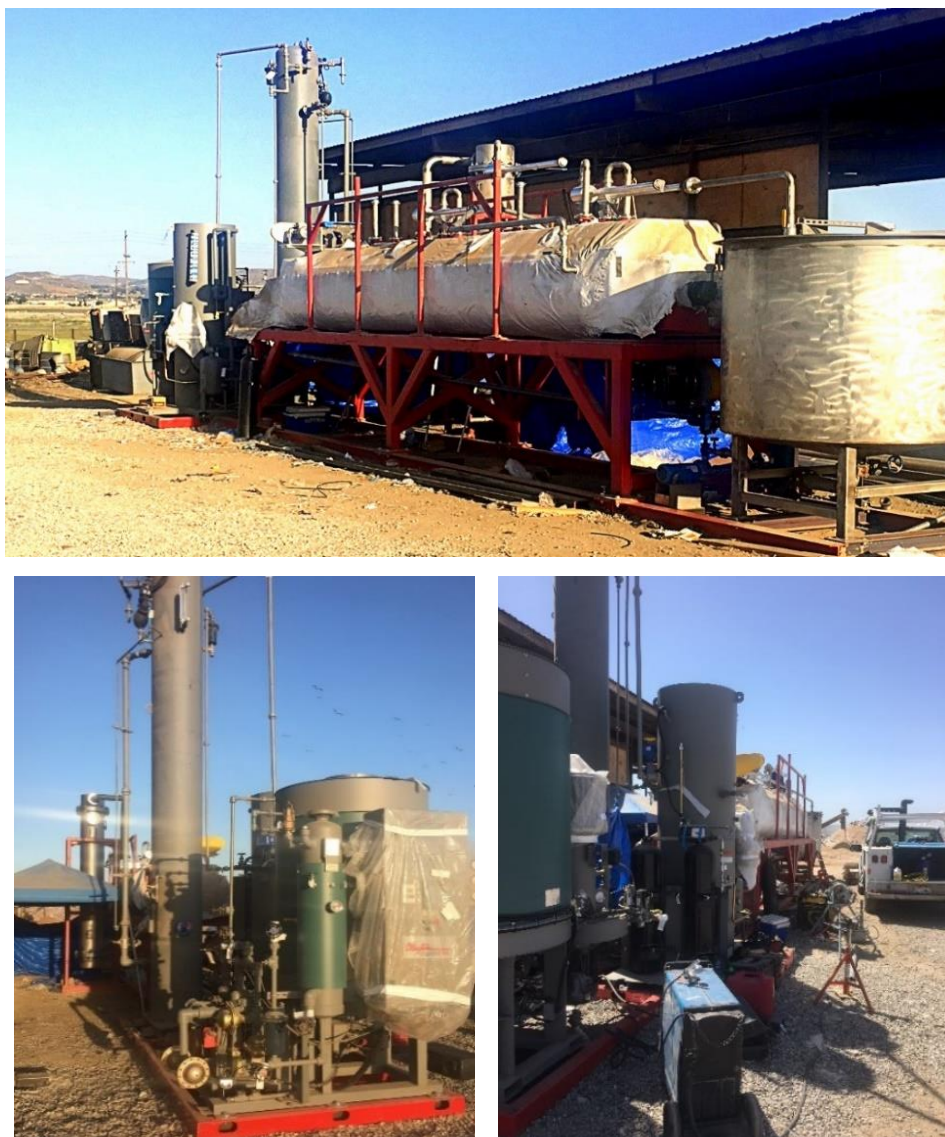
Figure 3.3: System Mechanical Installation at Martin Feed, LLC in Corona, California (GTI)
