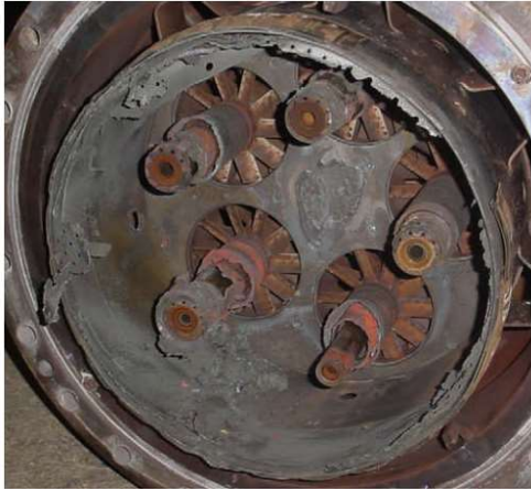
Figure I-5 burner assembly damaged by combustion instability [6]
