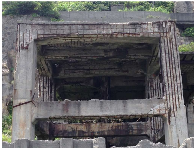
Photo—2.1 Deterioration in a RC structure
