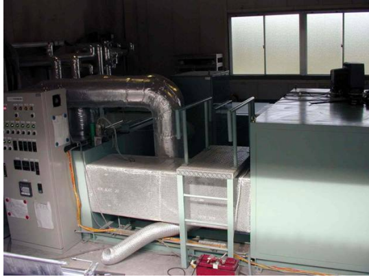
Heating/cooling capacity 5kW, installed in 1999
