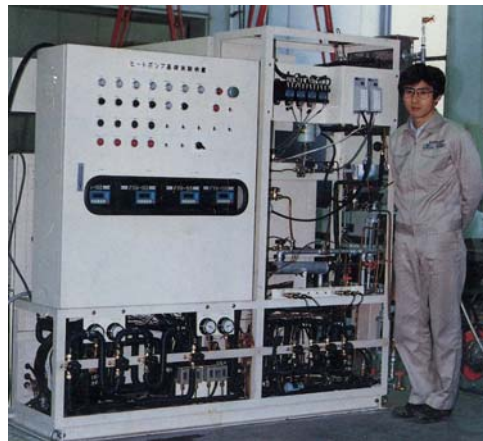
Heating capacity 4kW, installed in 1987
